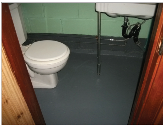
Poor Installation Sink Drain
