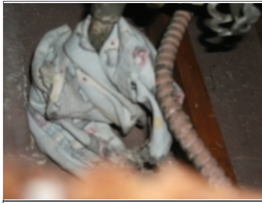
BX Cable in Ceiling Area
