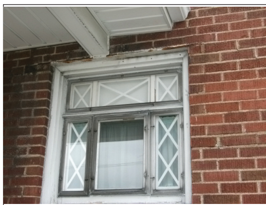
Window lintels and maintenance needed
