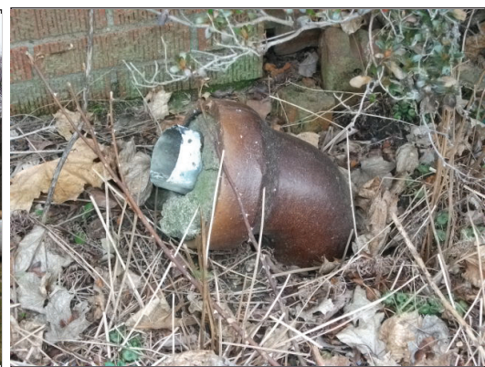
Garage broken loose leader
