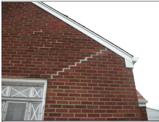
Repair attempt to brick.
