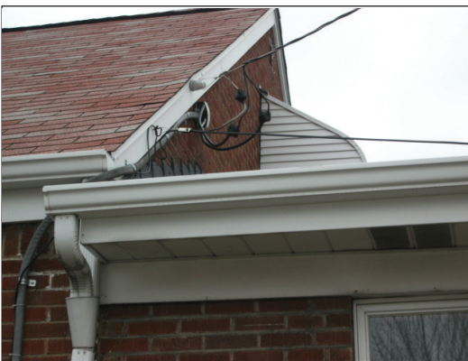
Poor clearance of electrical service entrance.
