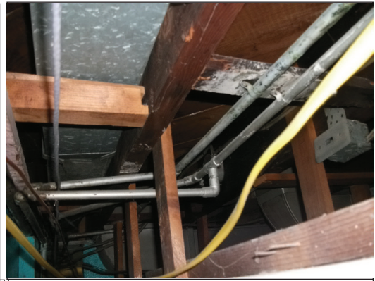
Hidden wiring electrical in ceiling.
