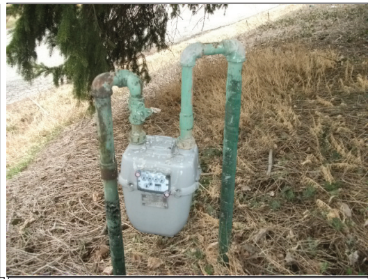
Gas Meter Near Street Rear
