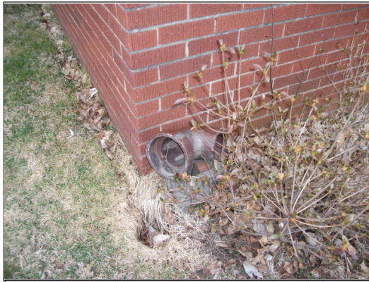
Garage Broken Loose Leader
