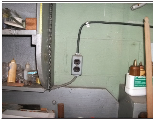
Electrical Outlet Garage
