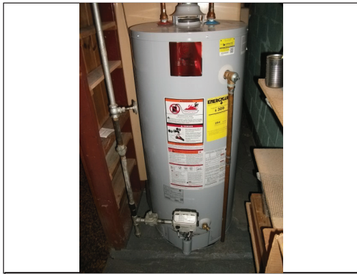
Hot Water Tank
