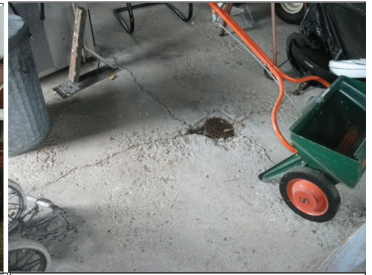
Garage Floor Conditions
