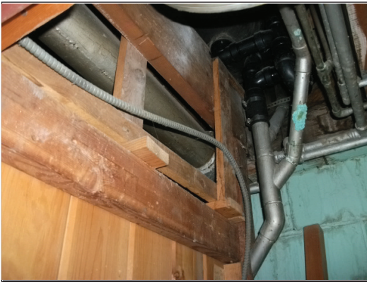
BX Cable in Furnace Area
