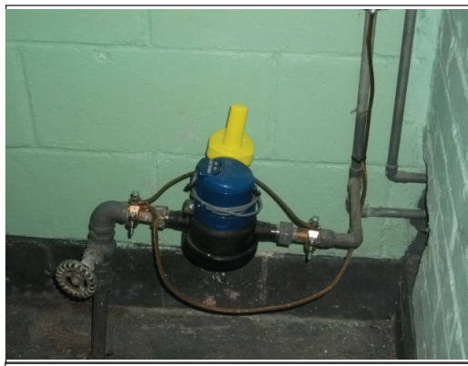
Electrical Ground on Water Meter
