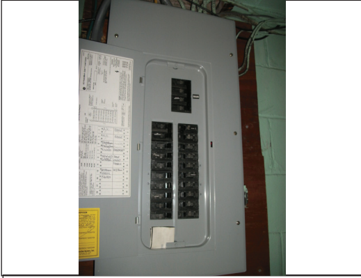
Main Service Panel & Approval
