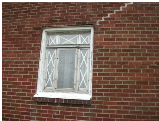
Damaged Lintel and expansion thru brick.
