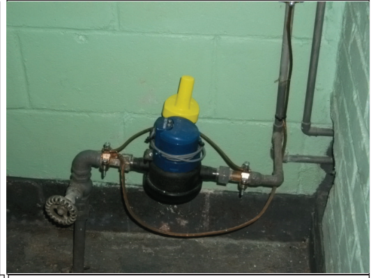
Grounding & Bonding Water Meter
