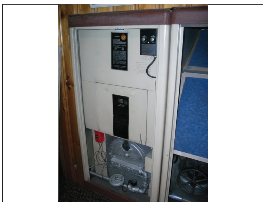
Front of Furnace Open
